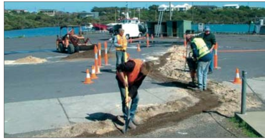
Workmen installing the surveillance equipment at the port of Robe, South Australia.
